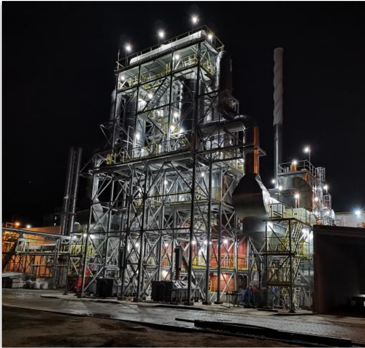
2x7 MW thermal oil boiler plant
